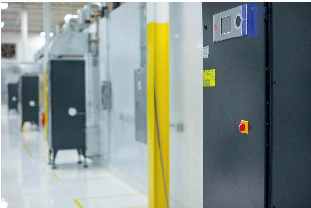
STULZ Precision Air Conditioners, deployed at Medicine Man Technologies, Inc. in Colorado
