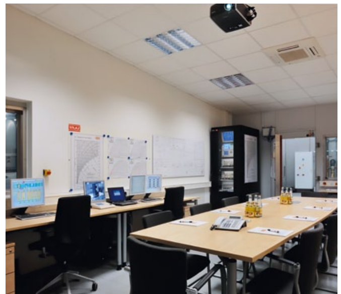
Experience the testing of your air-conditioning system live in our control room
