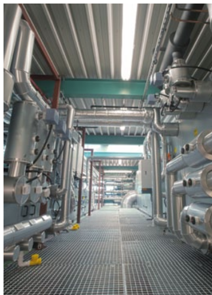
Pump stations for conditioning system
